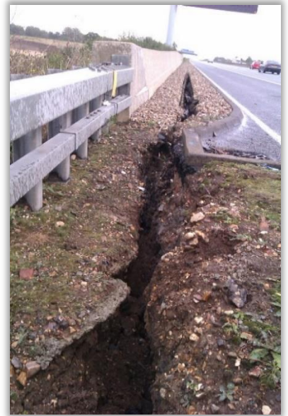
Crack in clay slope on M11 Source: HAGDMS
