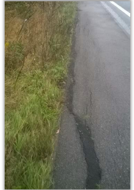
Shrink / Swell damage to A2, Canterbury, 2015. Source: HAGDMS
